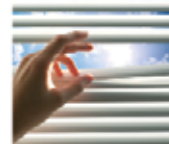
Automated solar shading and window blind control
